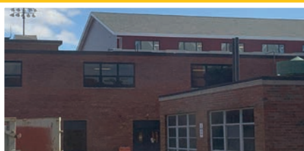
The old East Gym has been relocated to the second floor, requiring the ceiling/roof to be bumped up. Very exciting!
